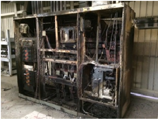
Fig. 2. Example of a damaged distribution cell due to high temperatures (Source:[4], accessed on 2022-02)
