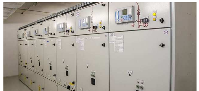
Fig. 1. Example of MV (Medium Voltage) switchgear with 8 (eight) cells (Source: https://electroalfa.ro/referinte-infrastructura , accessed on 2022-02)
